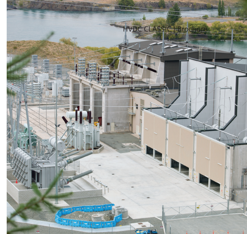
Benmore Power Station – the start of the Inter-Island link Pole 3
