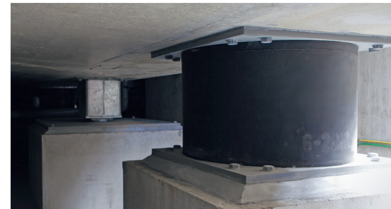
Seismic measures: rubber compensators for damping of vertical and horizontal oscillation of the complete valve hall/transformer foundation
